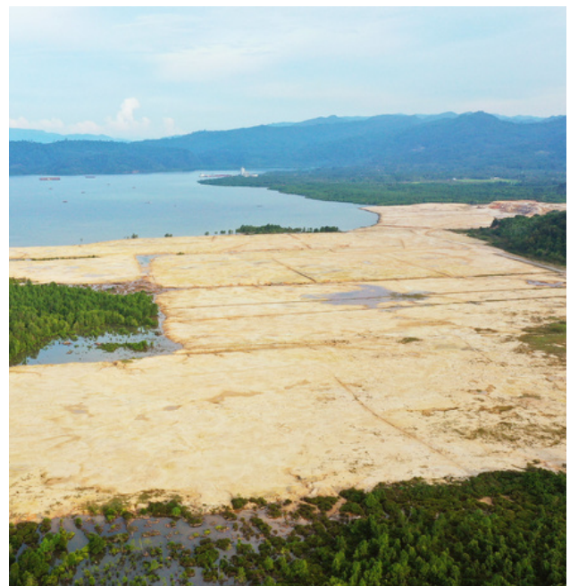
The PT Sungai Raya Nickel Alloy Indonesia (SRNAI) smelter is located in Landipo Village, Moramo District, South Konawe Regency, Southeast Sulawesi Province. This smelter is a National Strategic Project (PSN). Image credit: Courtesy of Yudi Nofiandi via Auriga
